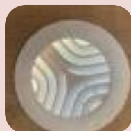
Lower ventilation grille
